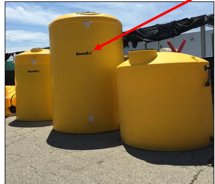
Aux. Storage Tanks
